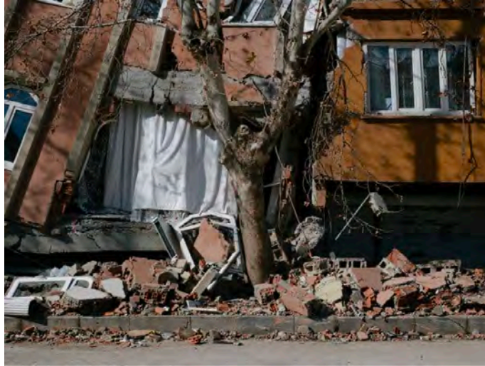
Damaged buildings in Pazarcik, Turkey. Emin Ozmen for The New York Times
