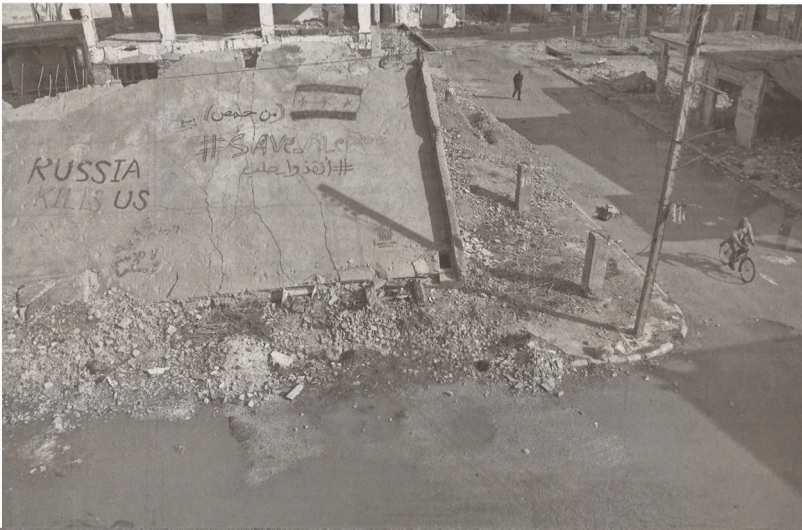
A collapsed building in Talbiseh, Syria. Egypt and Turkey are easing their positions on Syria as Russia asserts itself across the region to a degree not seen since Soviet times.
